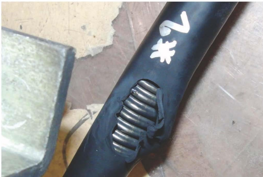
Fig. 4: High-current arc damage to jacket with undamaged tubing
